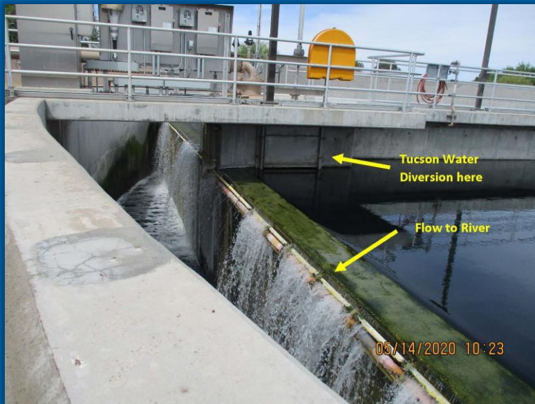
Downstream end of the chlorine contact chamber at Agua Nueva, Pima County Wastewater James Brown May 15, 2020 Image and caption used with permission
